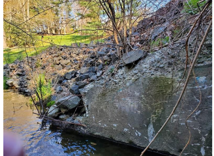
Upstream Wingwall – Deteriorated Concrete
