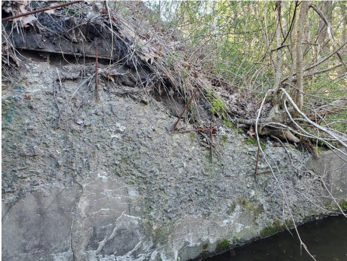
Downstream Wingwall – Deteriorated Concrete
