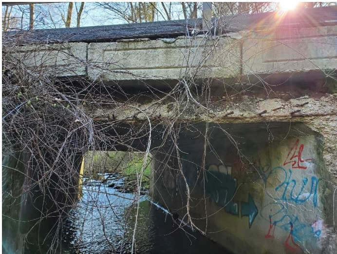
Spalling w/exposed rebar and section loss (typ)
