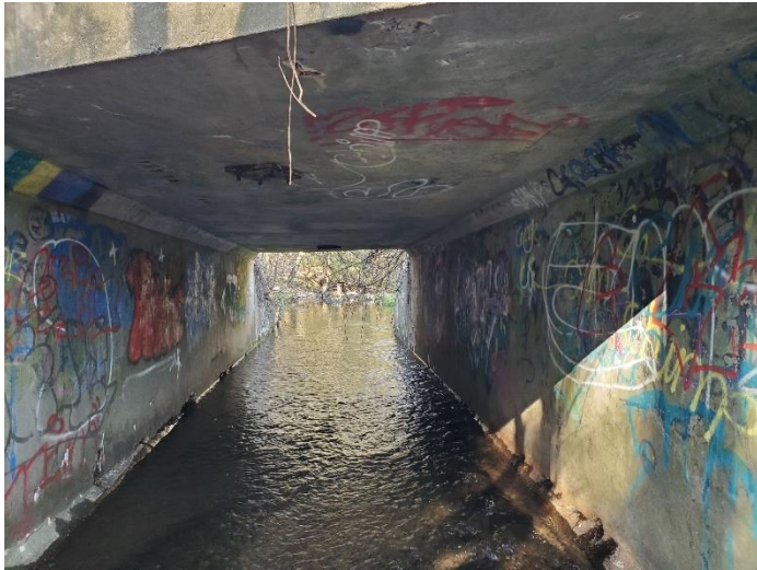
Downstream View – Scour / Spalling (typ)
