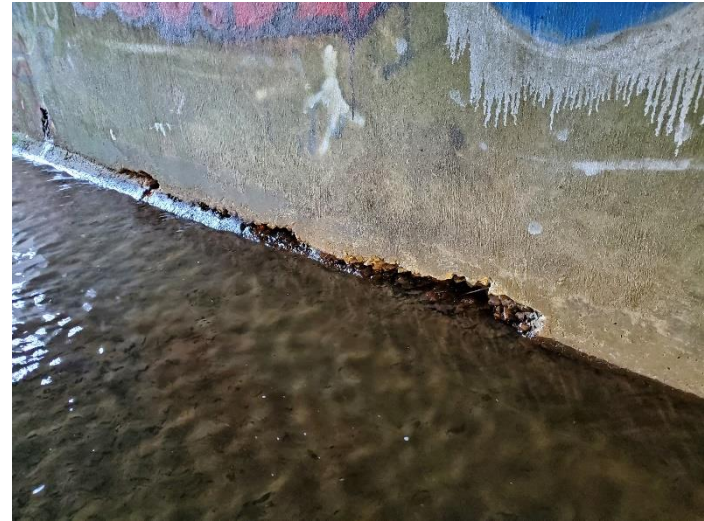
Stem at Waterline with exposed rebar w/section loss
