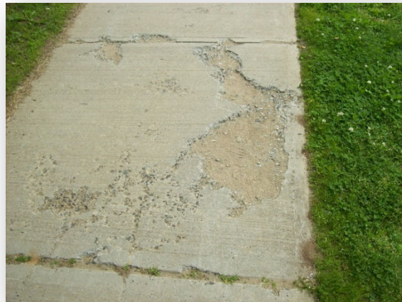
Sidewalk in need of repair
